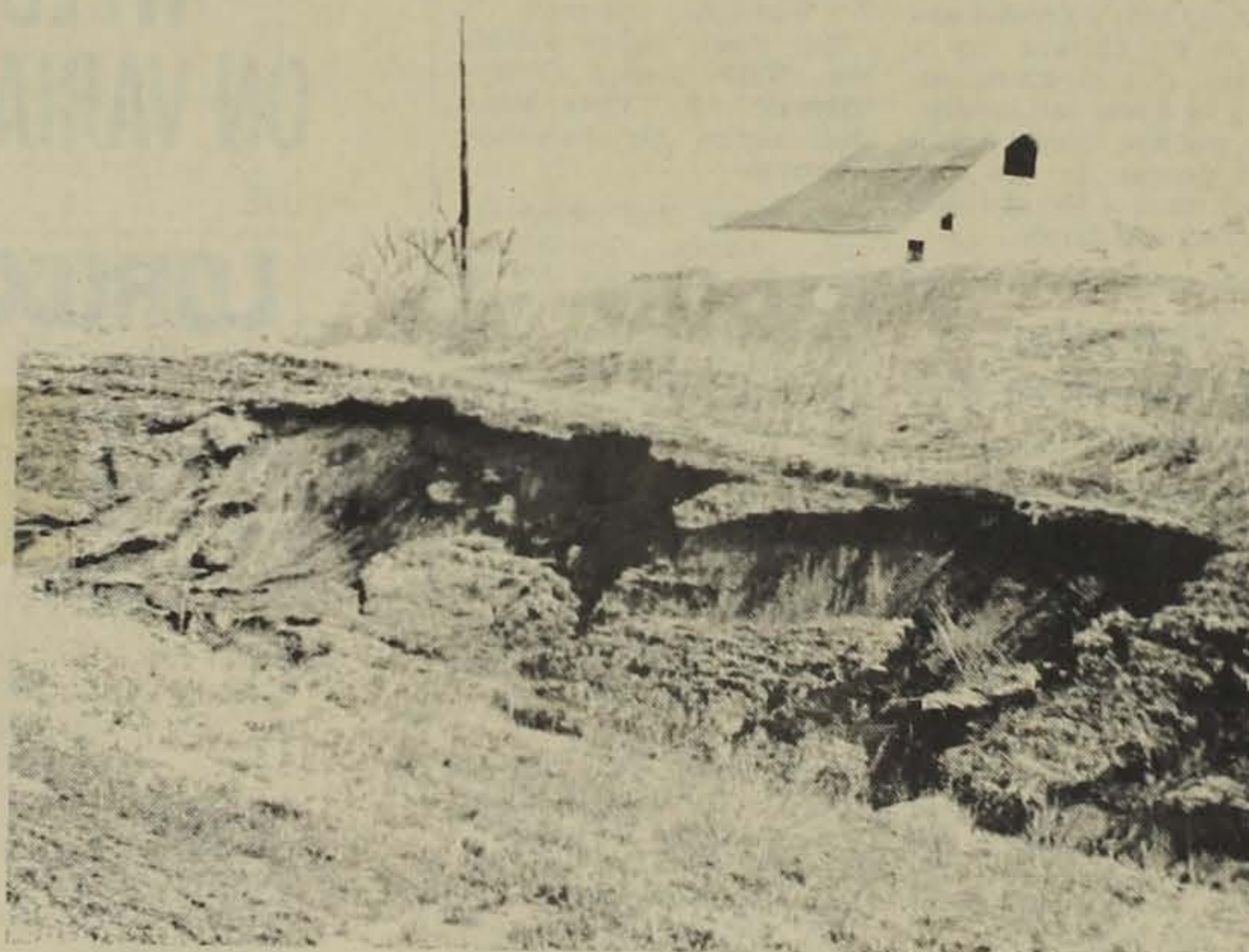
SUPER-SATURATED! Severe damage has occurred to road banks by soil sliding as shown in this picture taken near Murray along Highway 34. Damage has not been limited to new grading. Many banks along old roads have slipped also.
