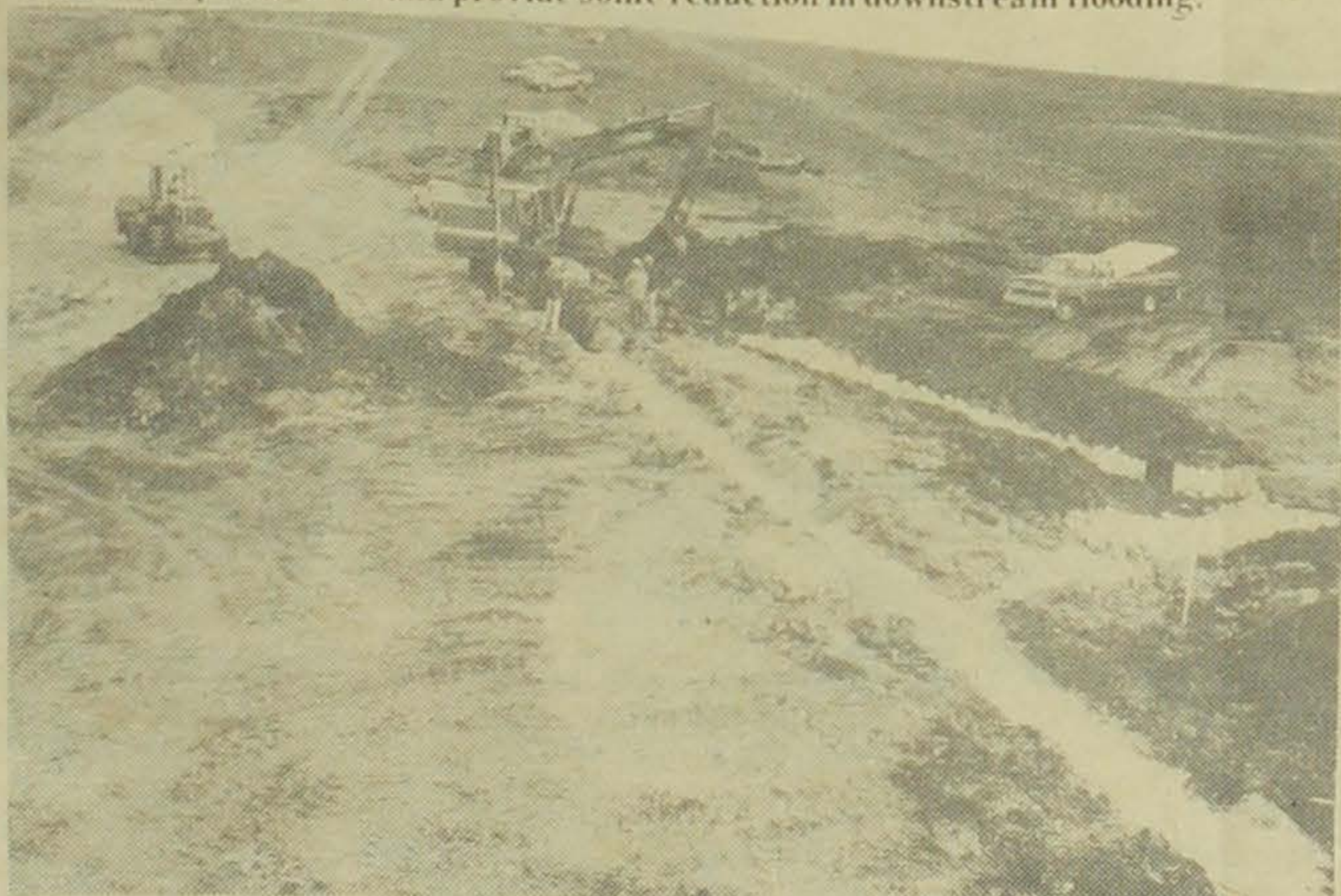
Important parts of a structure are the foundation drains made up of crushed rock. The drains are needed to carry away excess moisture in the dam to insure that the earthfill is stable and safe.
