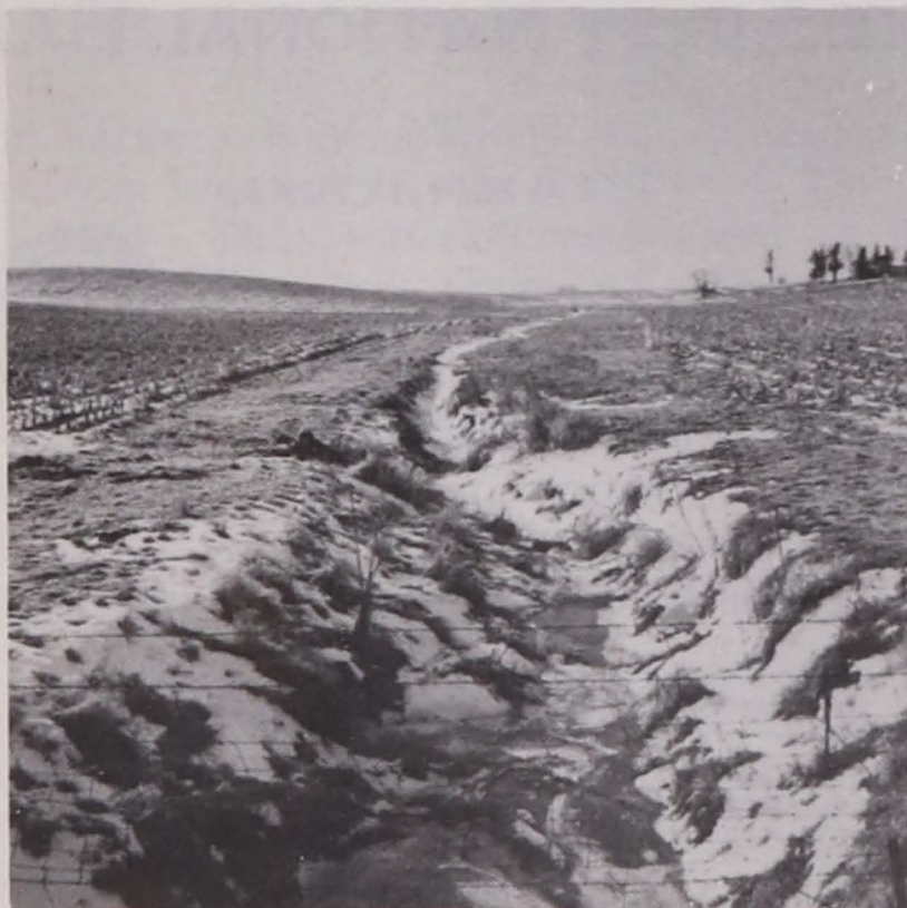
This photo shows an uncrossable ditch that is constantly cutting into the adjacent field. By reshaping and tiling this ditch it could be made into a grassed waterway --
