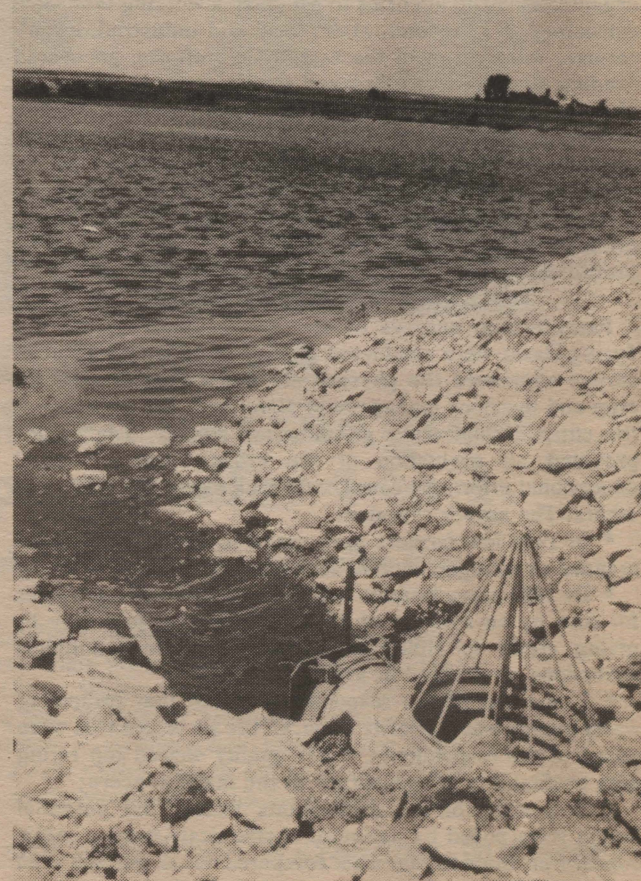
WATER LEVEL REGULATED — This structure was installed by Buchanan County on the pond at the Koutney Pond/Hoffman Woods located off Interstate 380, south of Brandon. The structure helps regulate the water level of the pond. Those involved in the building and design of the pond were the Soil Conservation Service, Buchanan County Road Department and Buchanan County Conservation Board.
