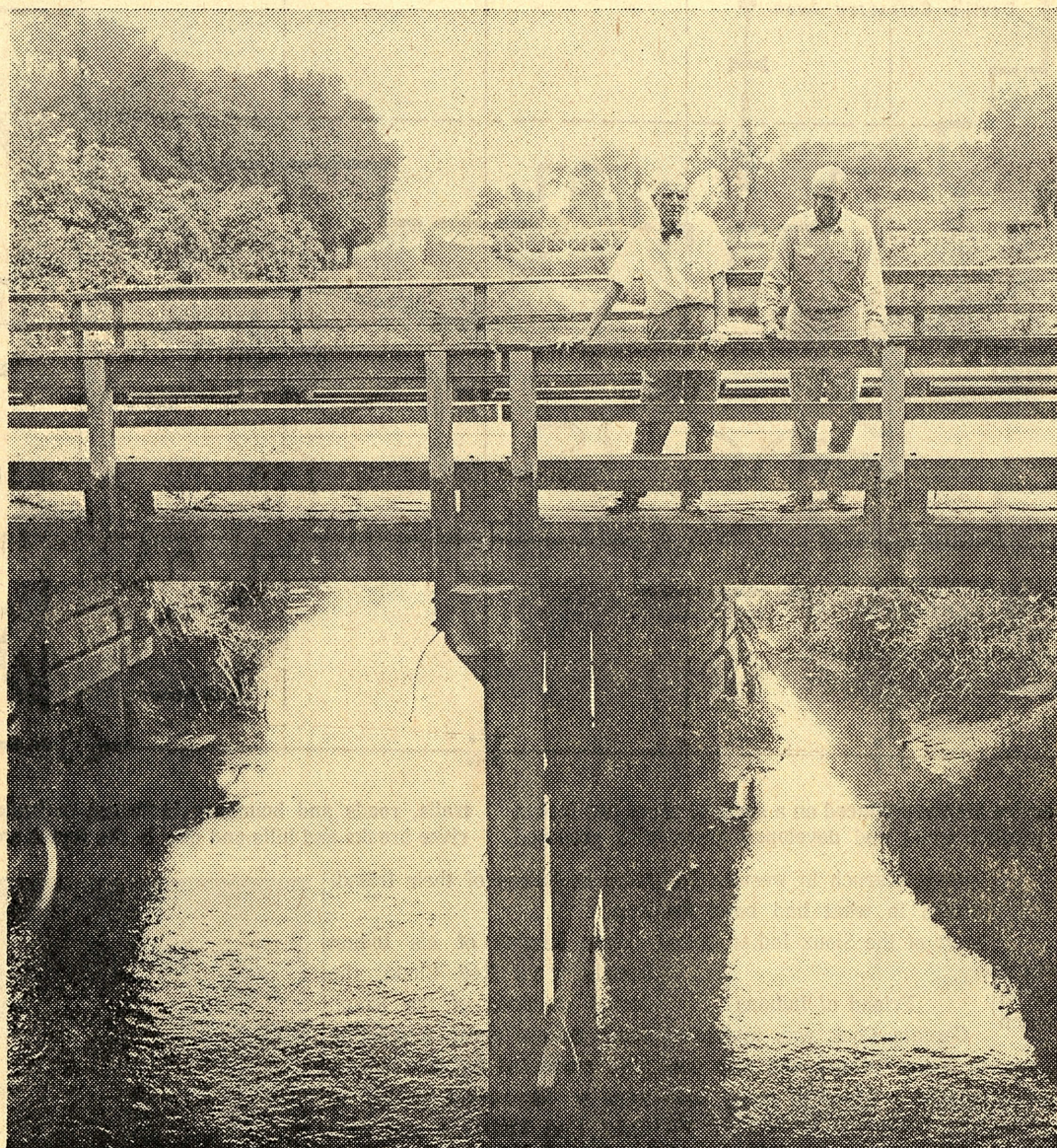
One of the bottlenecks partly responsible for Ida Grove's flood woes is this old wooden bridge, located over Odebolt Creek on Moorehead Ave. in the northern portion of the city. Another bridge to be removed (on Washington Ave.) is pictured in the background.
