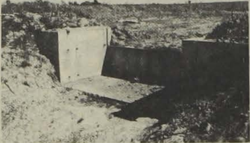
Grade stabilization structures can also be made of concrete as shown by this structure built on the Elvin Harms farm, Steamboat Rock.
