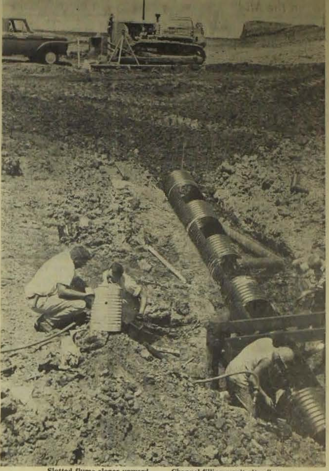
Slotted flume slopes upward . . . Channel filling won't alter flow.
