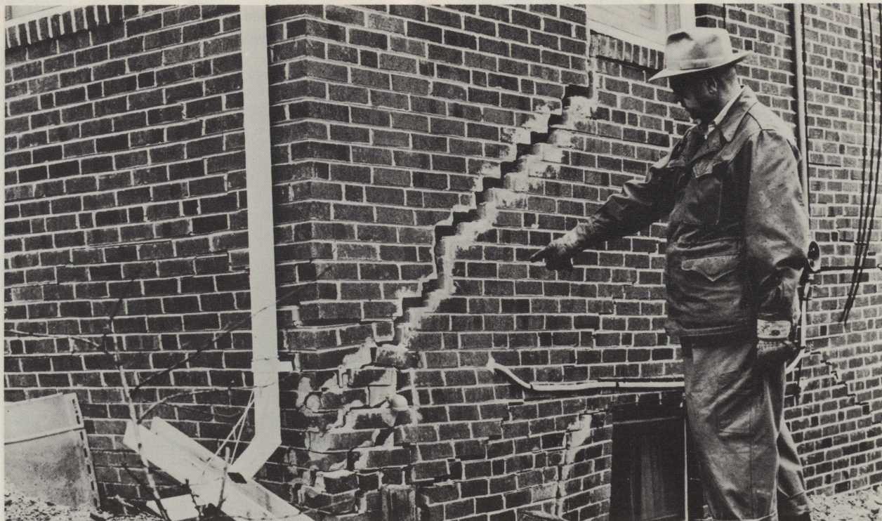
BN12938 This house was built on an unstable soil. The soil's swelling and shrinking with changes in the weather made the wall crack.
