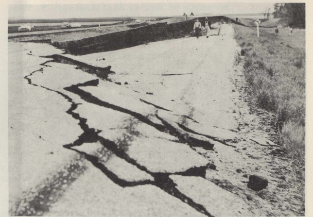
ND-603 The soil under this highway, built on a slope above the Red River, was unable to support the pressure. The highway could not be repaired and had to be reconstructed 150 feet further from the river.
