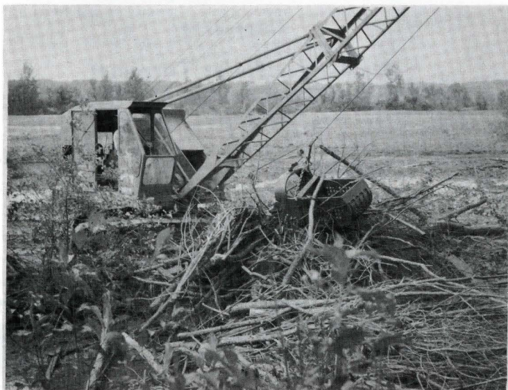
Clean up - After the Flood receded in the Tama bottoms. Rex Mackey is shown cleaning debris from an open ditch on the General Investment Co. farm.
