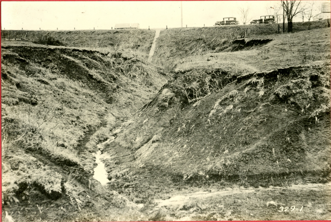
A large raw V-shaped gully carrying highway water that was steadily and rapidly growing bigger, deeper, and more active until 1930 when steps were taken to stabilize it.
