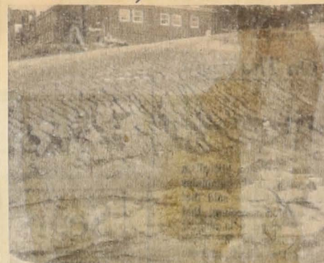
Eroded freeway area off High east of Third
