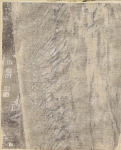
Eroded freeway area off High east of Third
