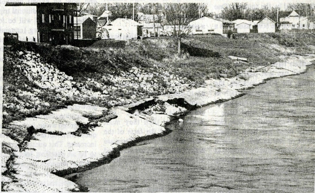
These concrete pads were installed north of the Iowa 99 bridge to inhibit erosion. They have deteriorated and will be replaced.
