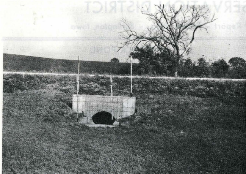
Drop box on road cuvert, serves as tile outlet and grade stabilization structure at lower end of long grassed water course on Mrs. Martha Schwaller's farm in Washington Township, operated by Leonard Calgren.
