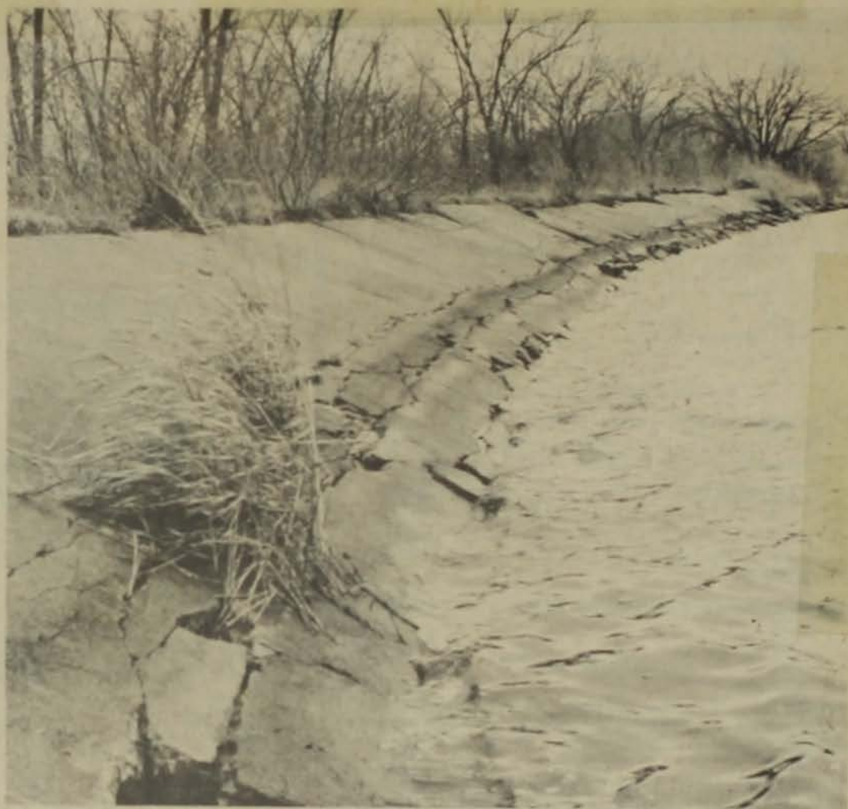
OLD SPILLWAY CRACKING UP: The present spillway at the East Lake dam shows evidence of cracking and shifting. Clarke County Conservation Board plans specify the removal of the concrete spillway and installation of a new spillway of precast reinforced concrete pipe with a
