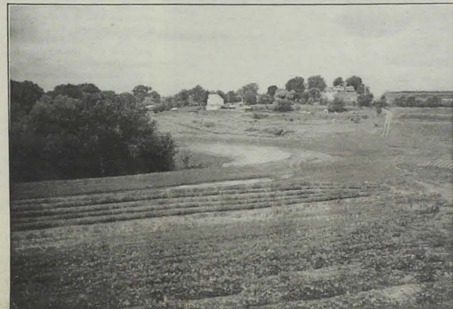
This completed terrace on the Dimon farm was especially designed to not only control the gully which had been seriously encroaching, but also provide roadway access to the fields beyond the structure.
