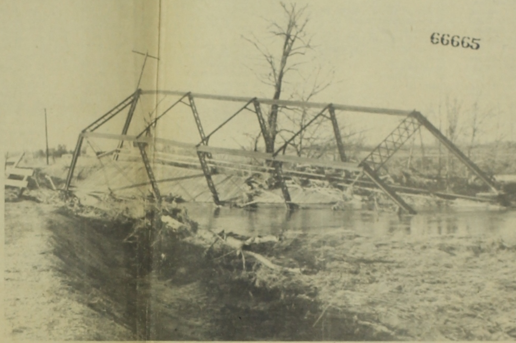
A bridge over 100 feet long was washed off its foundations following rains measured unofficially over seven inches
