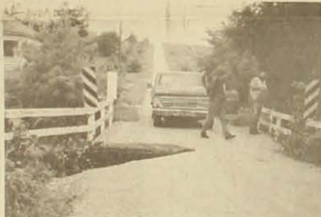
BRIDGE ISOLATED: Chris Smith and Harry Palmer stand on a bridge east of the Woodburn Cemetery. Note the gaping hole caused by erosion to the approach of the bridge. Clarke County road crews have been battling to keep county roads passable. County Engineer Rich McKnight said the workers are doing the best they can under difficult circumstances.
