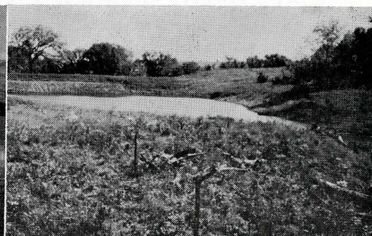
Delbert Calhoun and Clarence Hiner farms, Iconium Watershed, southeast of Iconium. 15 inch pipe drop-inlet gully control structure controls 52 acres of drainage and reduces run-off rate 70%. Water pool provides 1½ acres pond plus 6 acre feet of temporary storage.
