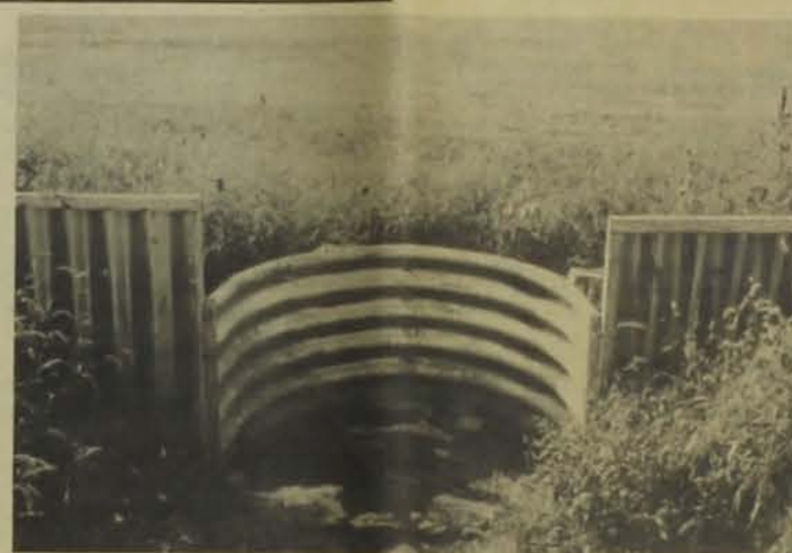
Erosion control structures are now built with reinforced concrete and sometimes with aluminum and concrete. Pictured is a gully control structure installed by Frank Cook of New Providence in 1979.
