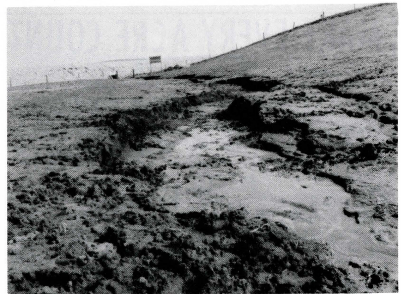
Rains and run-off in 1965 were rough on newly shaped waterways. This one will need to be re-shaped.
