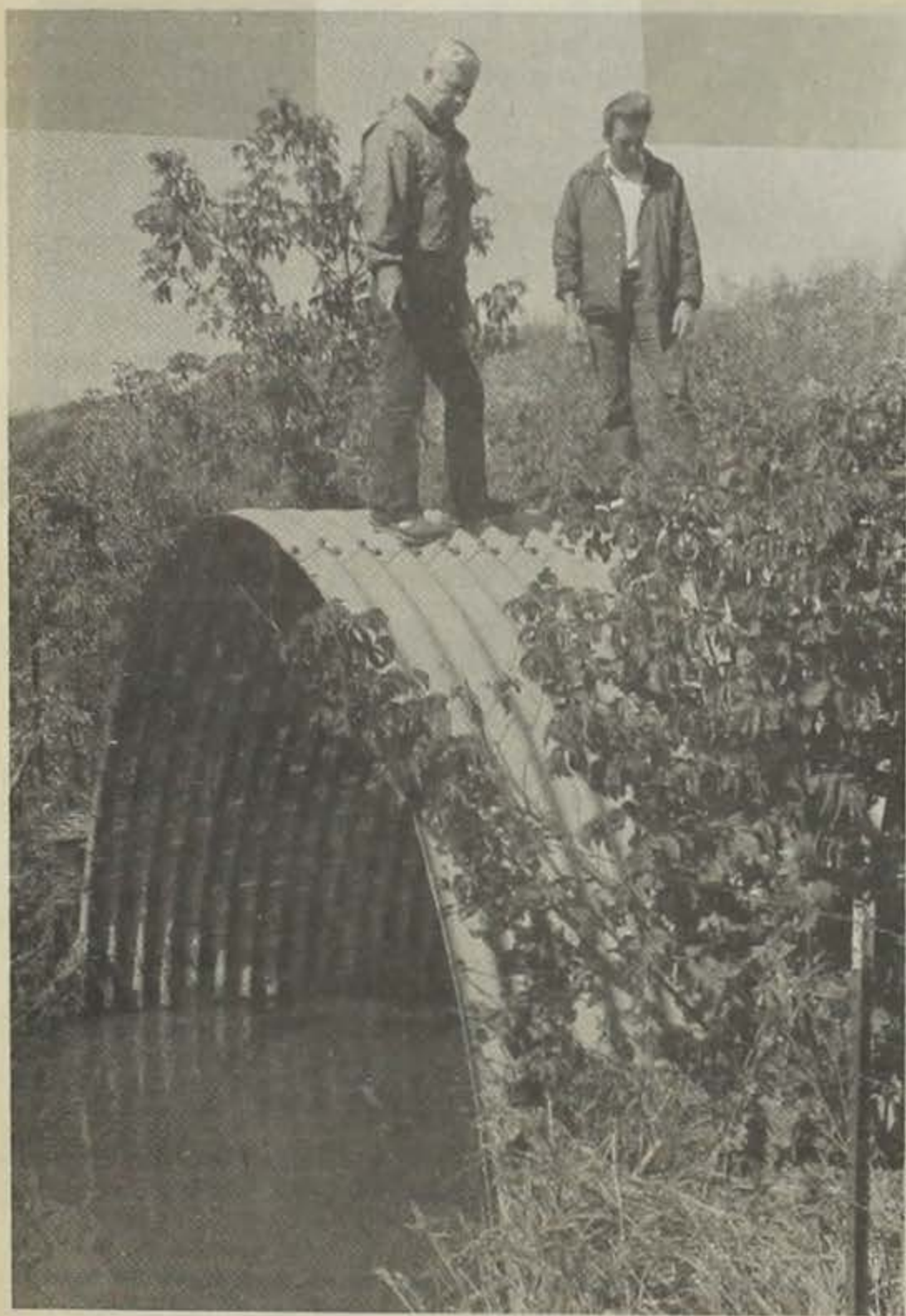
DAMAGE SURVEY: State Rep. Jack Beaman and Clarke County Supervisor Steve Smith survey the outlet of a 10-foot culvert damaged by flood waters. While the pipe appeared to be unscathed from this end, the inlet (see picture at right) presented another story.
