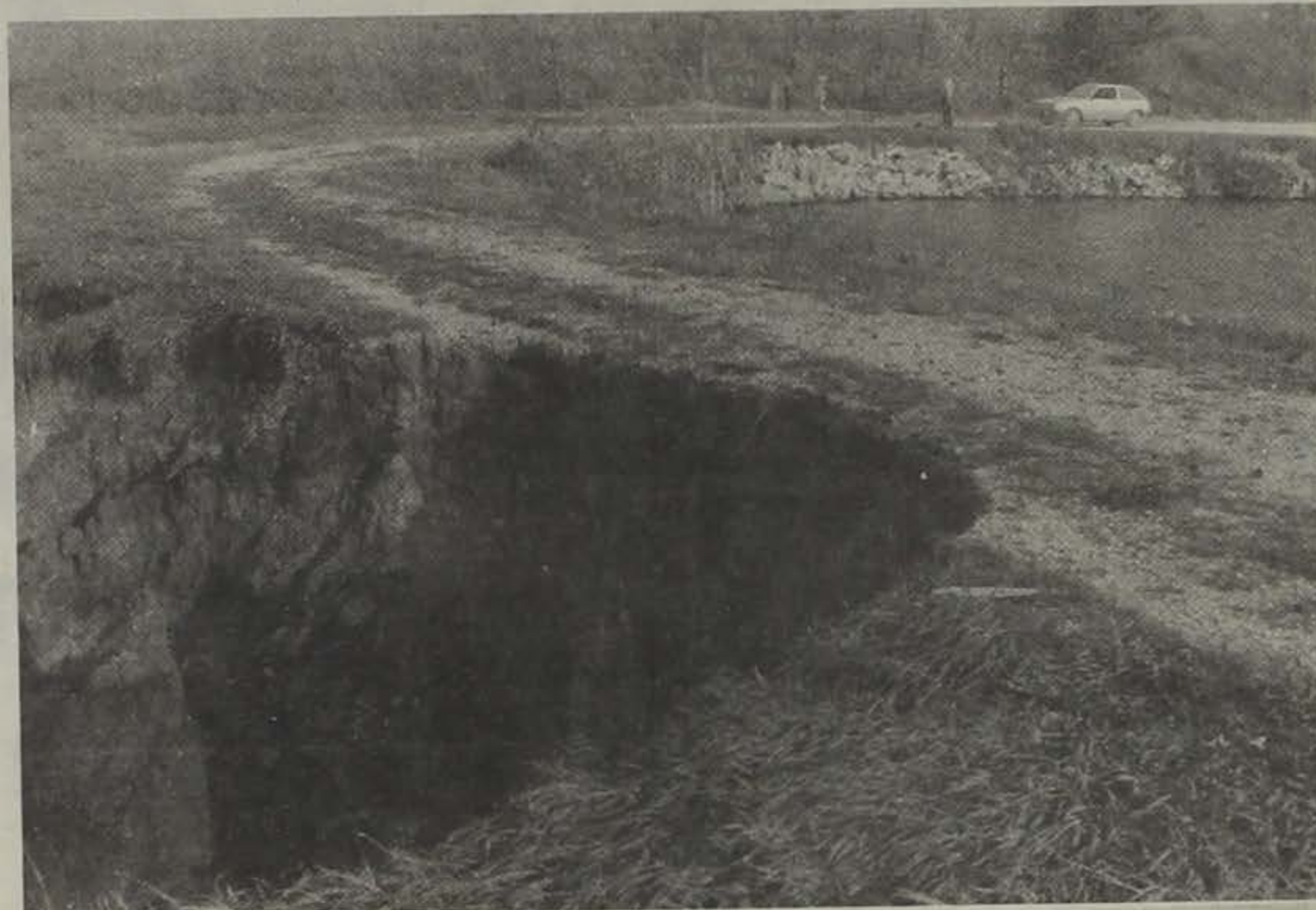
A BIG BITE: September floods washed out large portions of the backside of the Q-Pond dam. The dam, damaged in 1987, was repaired at the time with materials the state now considers unsuitable.
