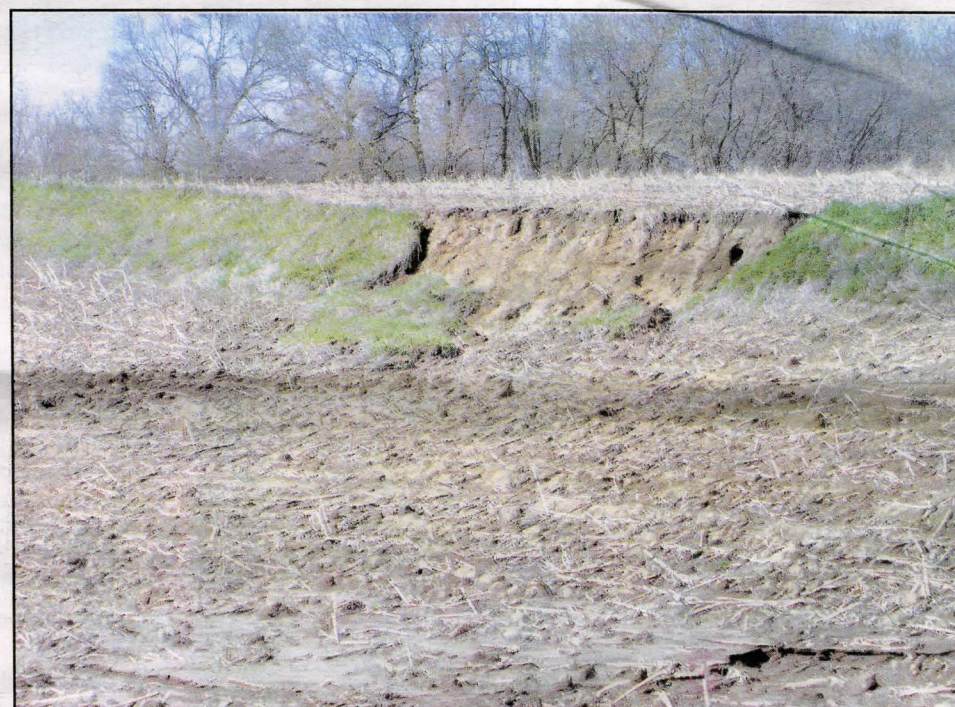
Grass back terrace, southeast of West Union, damaged during the heavy rains in the spring of 2008. The terraces were also weakened due to rodents working through them.
