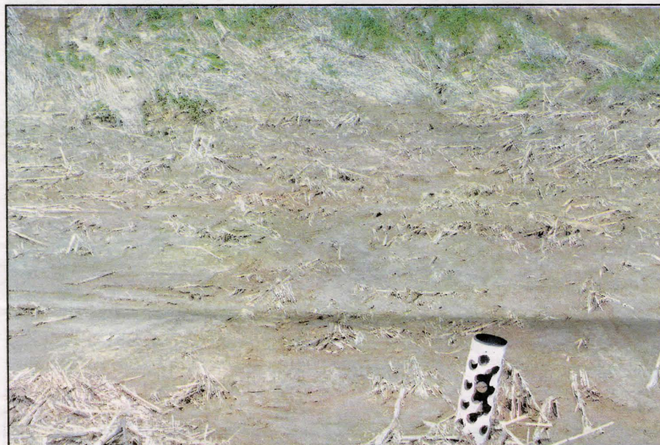
A terrace intake installed originally to approximately 3 foot in height. During the heavy rains of 2008, the siltation collected at the intake leaving the soil on the land. In order for this terrace to function properly, the storage area will need to be cleaned out and replace damaged inlet. Maintenance to terraces is important keeping terrace capacity, storage, ridge height and outlets to design. Control weeds, brush and trees to the back slopes/front slopes too for maintenance.
