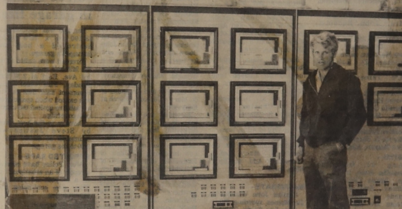
Hatchery biologist Andy Moore is shown with the control panel of the monitoring system located in the administrative office. If a malfunction occurs, an alarm is sounded and the panel can be checked to determine the problem and its location.
