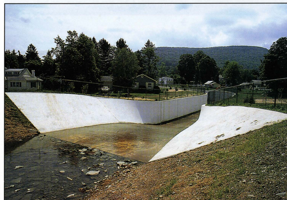
Left: Flood Prevention Channel.
