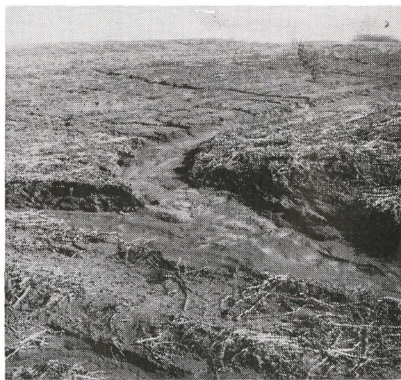
Terrace outlet finished improperly; no grassed waterway, shows high degree of soil erosion. Approximately six inches of soil lost in this channel; Cooper Creek Watershed.
