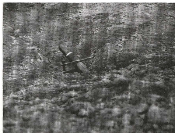
This is a typical picture of a propped outlet on a drop-inlet structure. These structures back water up over eroded areas and then during periods of excessive runoff, tend to step the water down through the structure and out of this type of outlet. As the water comes out of this, it will tend to cut a small "scour hole" which provides a shock absorber effect for the water as it is released on the downstream side of the structure.
