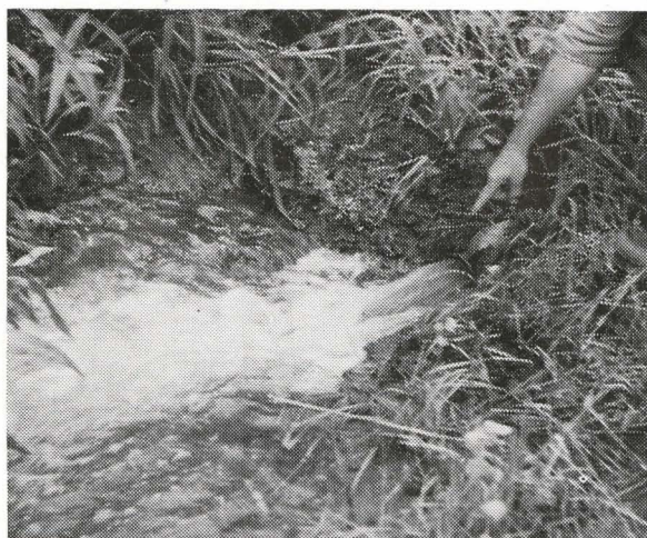
The outlet of a four-inch trickle tube in the John Mitchell farm pond, Cooper Creek Watershed. These trickle tubes are being used in several of the Appanoose County SCD ponds to help cut down the amount of water going through the emergency spillway on the farm ponds.
