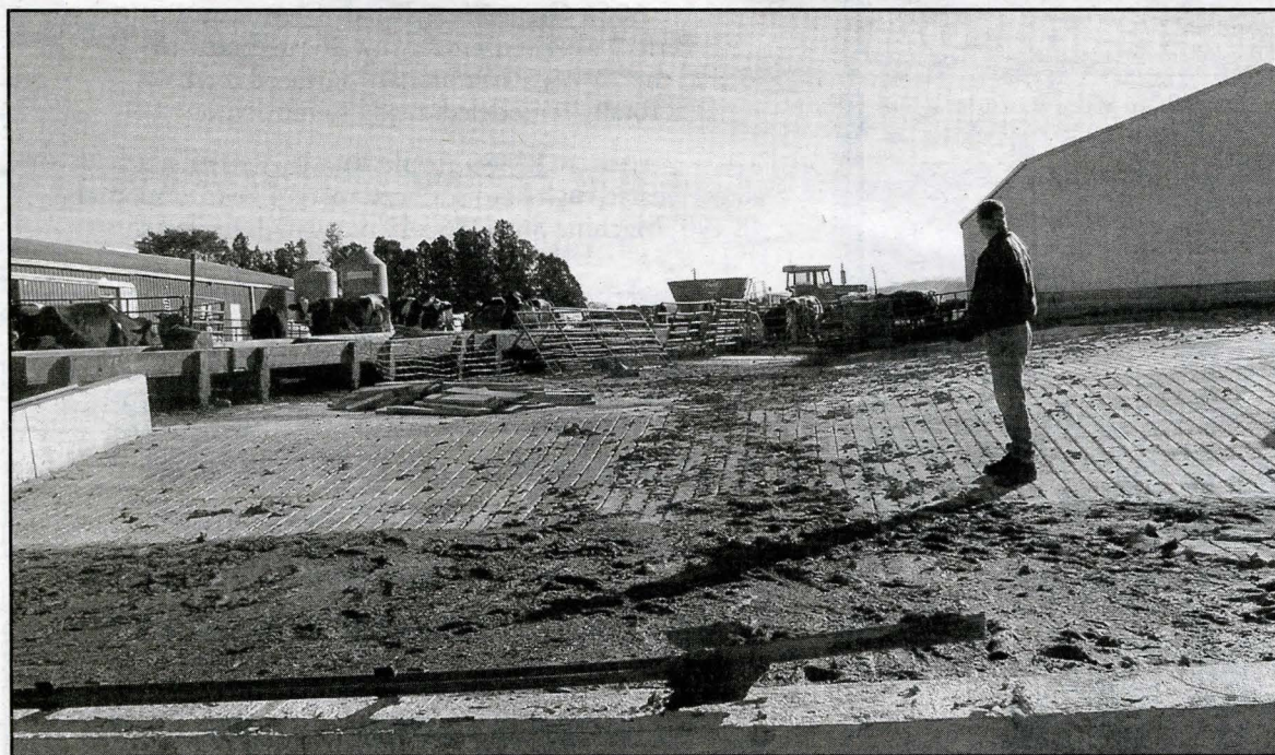
Mike Baumler's newly constructed settling basin and stacking facility. Mike has controlled 4370 gallons of water per one inch of roof run off with gutters and a diversion above the lot. This has made a tremendous amount of difference in the quantity of water running through his feed lot. Manure is captured in the basin and liquids are filtered in a grass channel. Livestock manure can be applied to cropland and utilized for their nutrients. This will cut Mike's fertilizer bill when he can take credit for the manure applied.
