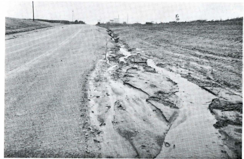
Critical erosion and sedimentation along public roads costs county taxpayers thousands of dollars in annual road repairs. In addition the dangers of washed out culverts and overturning farm tractors brings accidents and law suits to haunt the county government. On May 13, 1970, a 3 inch rain caused this extensive damage to a new road project in the Rathbun Dam area. Conservation officials estimate there are over five hundred active critical areas such as this on Appanoose County roads.
