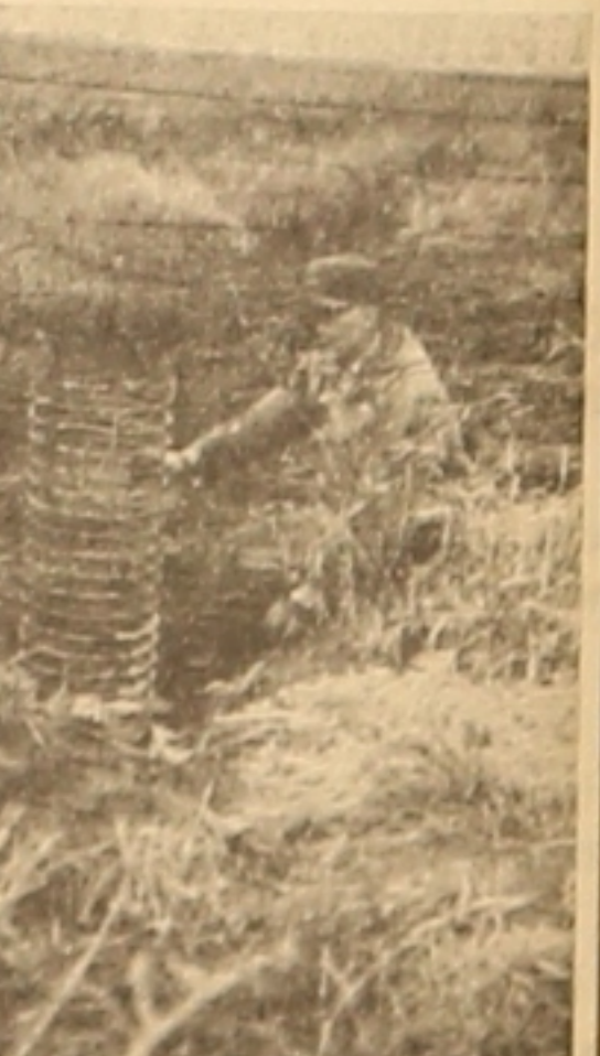
DALE WATSON is shown examining a surface intake which is part of a mutual tile system constructed in Putnam township. Watson, Albert Roepke, and W. R. Child formed a drainage group to get better tile outlets. The project included 8", 10" and 16" mains.
