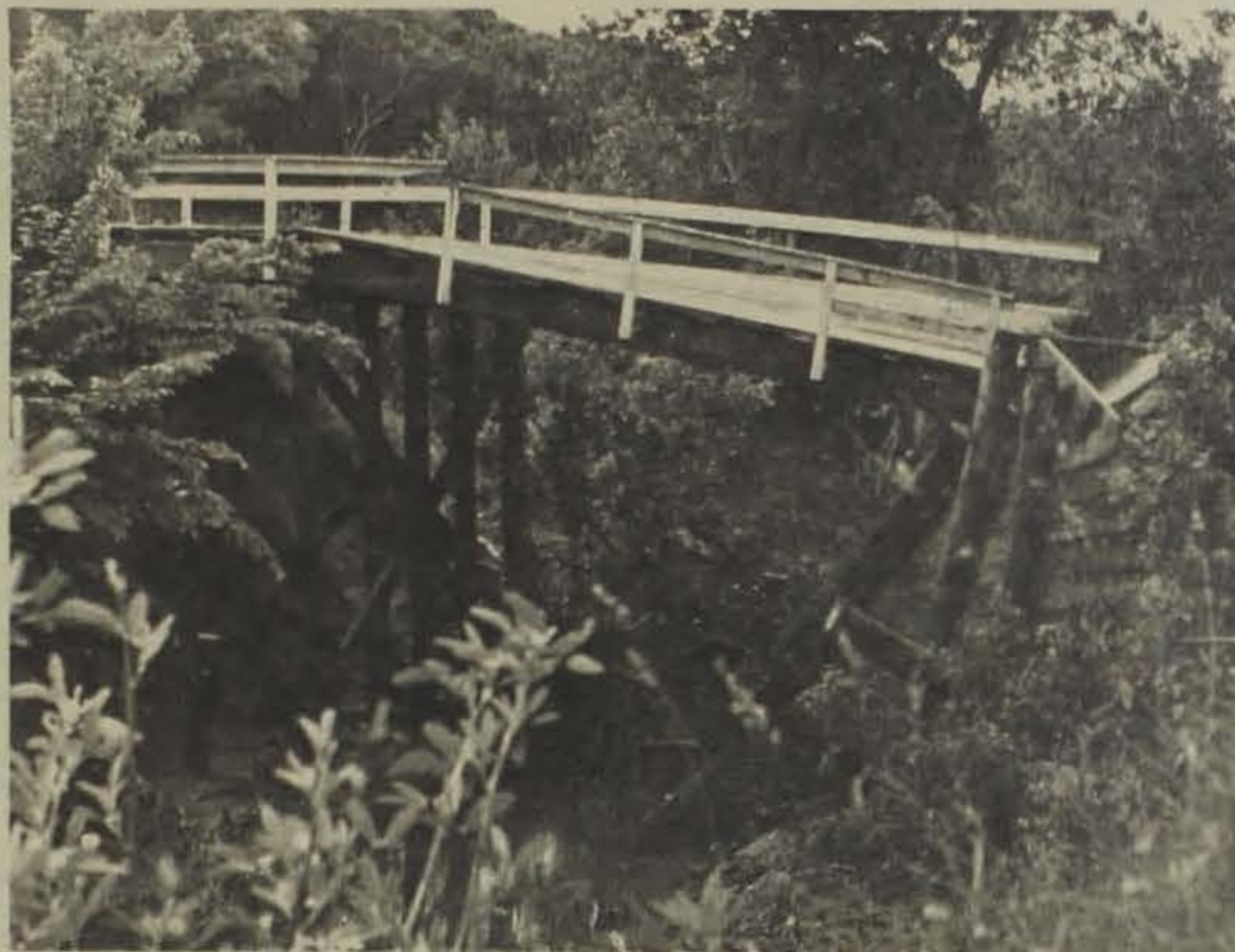
WASHED OUT: This 48-foot bridge on the Otto Huss farm northeast of Osceola was one of the county bridges that succumbed to high waters over the weekend. The bridge spans
