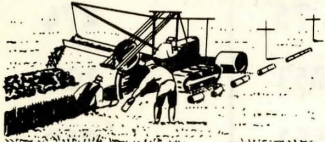
Tile drains 667 miles
