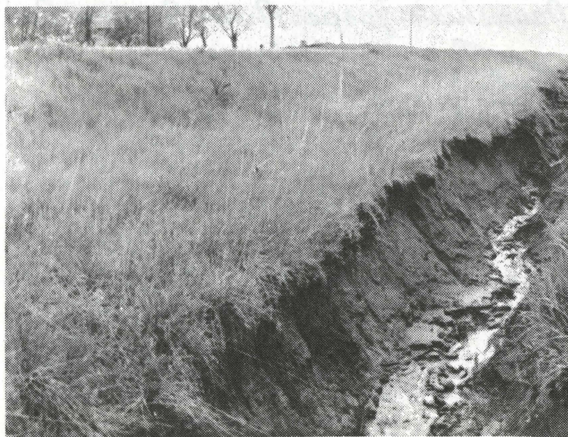
Unprotected road ditches eroded badly from May and June rains.
