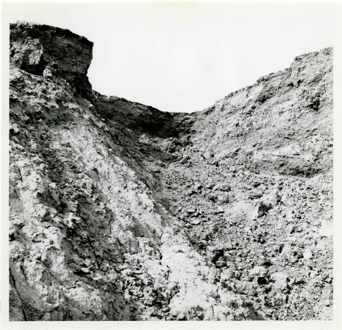
AN EARTH SLIDE OF THE POND FILL-ONCE THE LOWER PART OF THE FILL HAD WASHED OUT.
