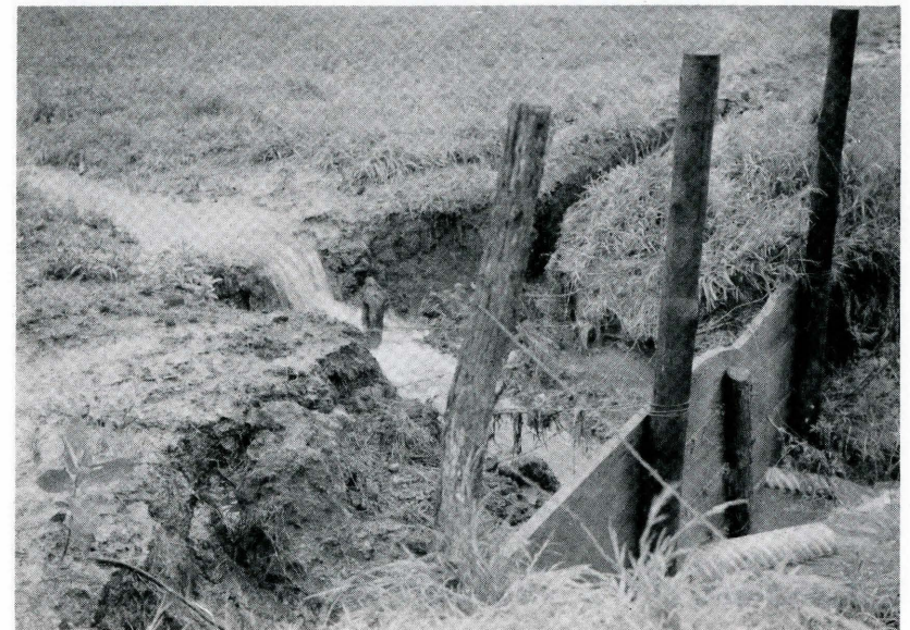
Improvised plank dam--inadequate for waterway or tile outlet. Note two culvert pipe tile outlet in lower right.
