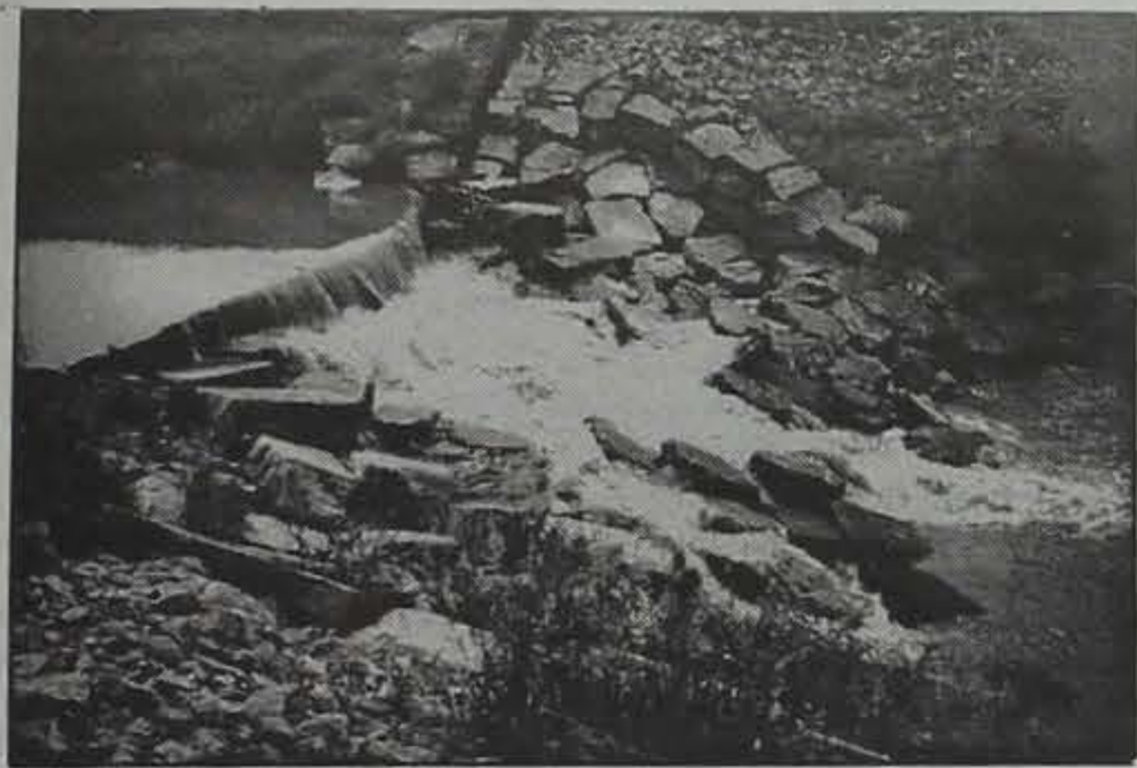
This structure has been controlling the flow of Mosquito Creek for 26 years. Many more of its kind are needed, but funding is difficult to obtain.
