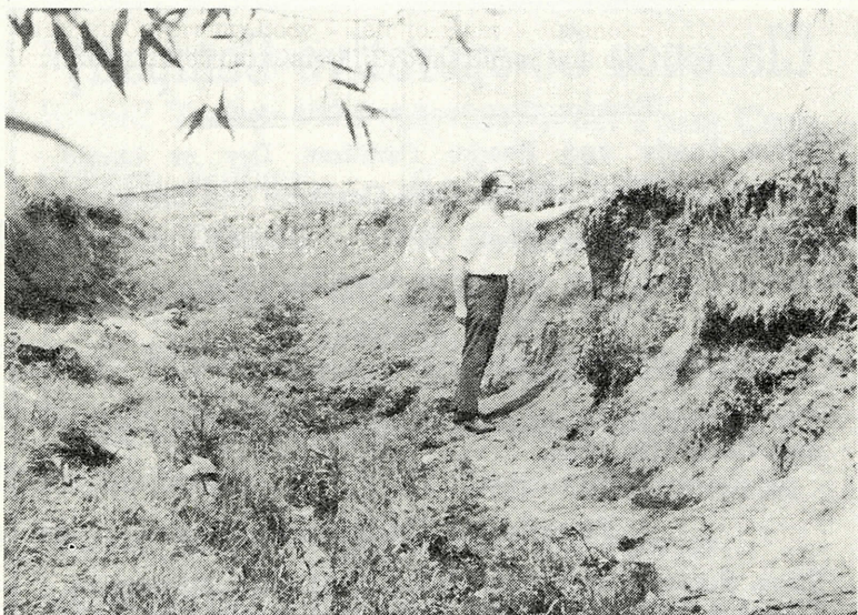
Don Williams observing a gully on the Harold Barnhart farm. This problem was solved late in 1971 with a structure and a good grass waterway.
