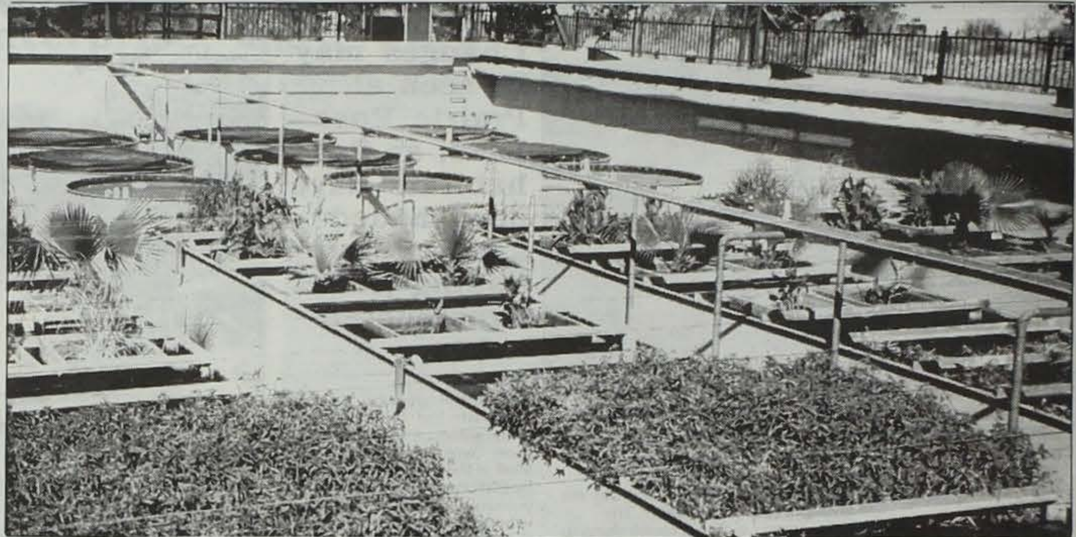
These large tanks are part of the wastewater treatment system at the Ethel M. Chocolate Factory. Growing plants have transformed the site into a thing of beauty.
