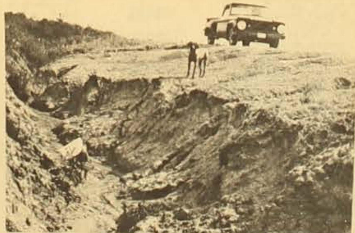
Erosion in the county road ditches is a serious and widespread problem in the county. A survey of the county roads to locate serious erosion areas is being conducted. With
