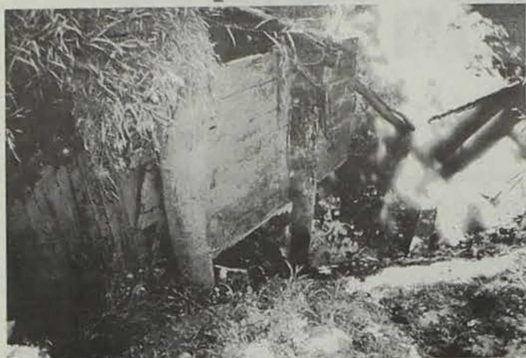
This photo, taken in 1997, shows the degradation of the streambank, and also the deterioration of the old wooden flume.
